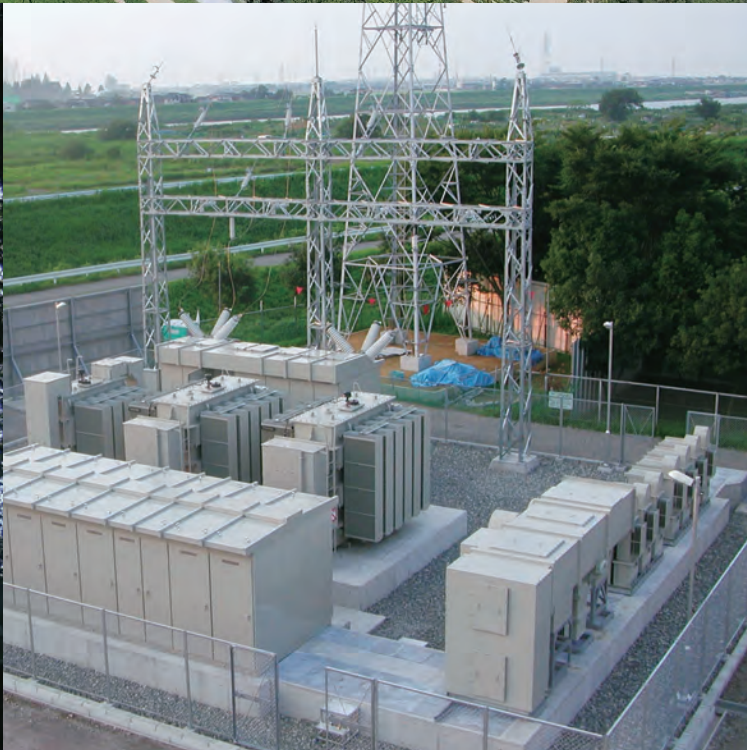
青森県 Wind Farm Tsugaru "Green Power Investment" (Top photo) Power Supply System Aomori Pref.
