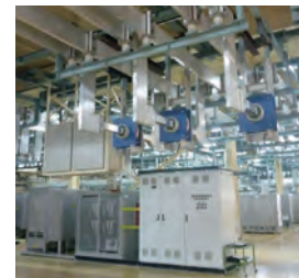
■量子科学技術研究開発機構 JT60SA 電力設備 茨城県 JT60SA National Institutes for Quantum and Radiological Science and Technology Power Supply System Ibaraki Pref.
